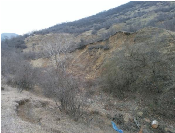
Photo 1: The general view of erosion-landslide genesis debris flow tributary Jokhtaniskhevi drains and its adjacent degraded slope
