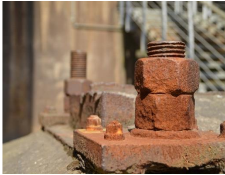
Image 1: Some corrosion phenomenon
