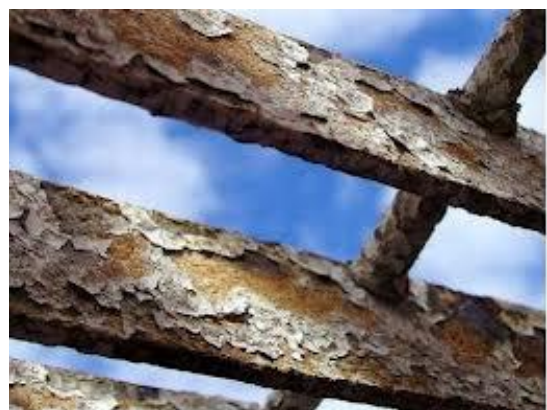
Image 3: The chemical-electronic corrosion
